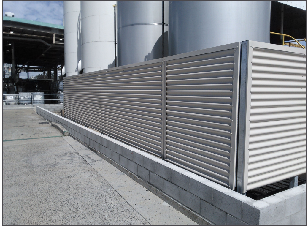
Engineering design of bund storage and screen protection plus site inspections for new Intermediate Bulk Container (IBC) storage facility.
